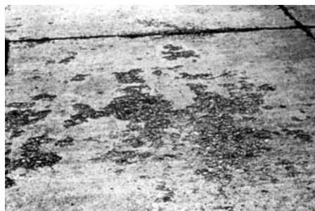
Fig. 3 Freeze-thaw cycles can cause scaling of concrete surfaces as shown on this pavement.
