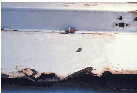
Fig. 2 The area of the same carbon steel pipe system as in Fig. 1 where the heater clips were placed in direct contact with the pipe, without insulation. This caused overheating because the pipe was in direct contact with the steam heater. The combined effect of waterline attack and elevated temperature is the cause of failure.
