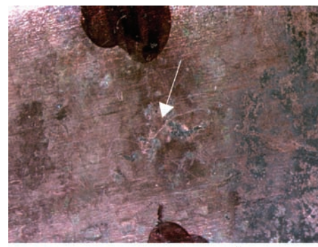
Corrosion form and mechanism Localized corrosion, pitting, formicary corrosion Material Copper Product form Evaporator coils; heating, ventilation, and air conditioning
