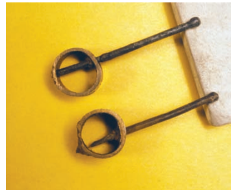
Corrosion form and mechanism Metallurgically influenced corrosion, galvanic Material Carbon steel and copper Product form Copper water tube
