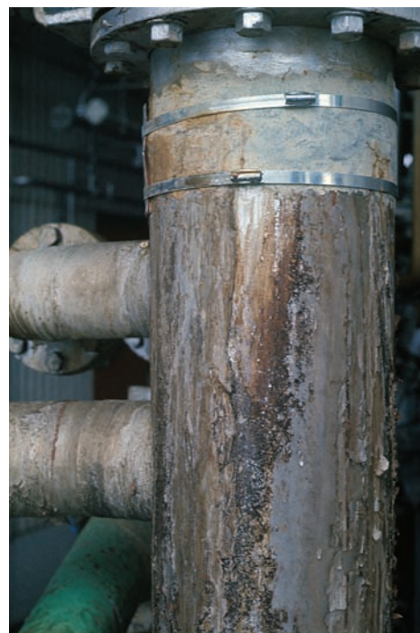
Corrosion form and mechanism Environmentally induced cracking, stress-corrosion cracking Material Type 304 stainless steel Product form Water supply pipe
