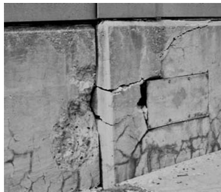
Fig. 4 Typical indicators of alkali-silica reactivity are map cracking and, in advanced cases, closed joints and attendant spalled concrete.
