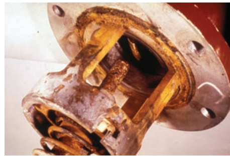
Corrosion form and mechanism Metallurgically influenced corrosion, galvanic corrosion Material Cast aluminum alloy and brass fittings Product form Drain valve from road tanker
