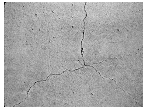
Fig. 6 Restraint to drying shrinkage is the most common cause of concrete cracking.
