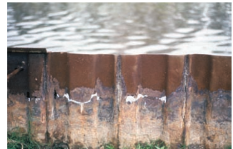
Corrosion form and mechanism Underdeposit and waterline attack Material Galvanized steel Product form Piling for canal bank
