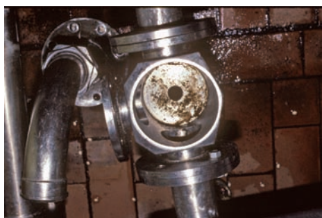
Corrosion form and mechanism Pitting, underdeposit attack, crevice corrosion Material Process pipe connector Product form Type 304 stainless steel
