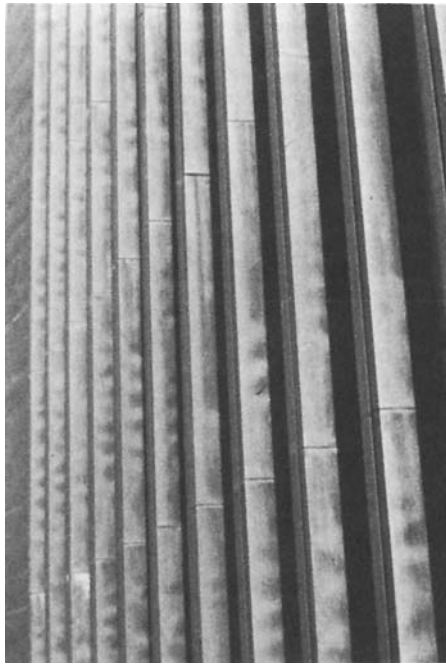
Fig. 12 Clad columns with less than 18-gage cover, resulting in oil canning
