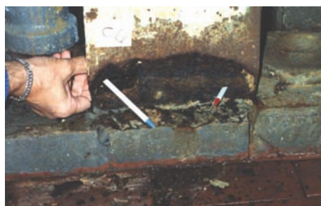
Corrosion form and mechanism Uniform corrosion, atmospheric Material Steel Product form Steel column
