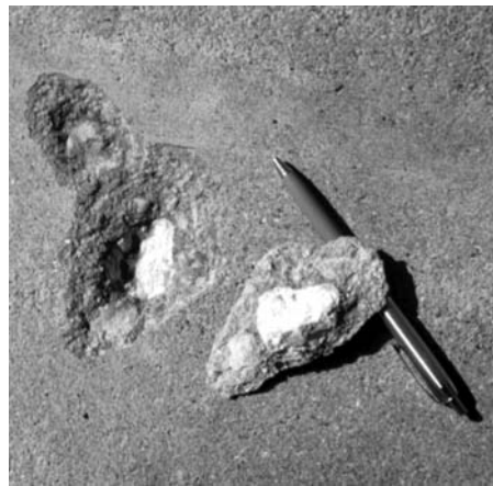
Fig. 8 Some aggregates absorb water and, upon freezing, expand to produce a popout.
