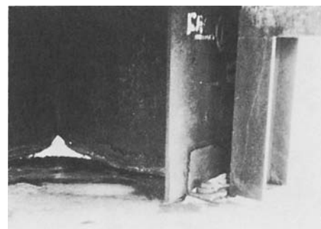
Fig. 10 Formation of lamellar rust due to moisture wicking upward from beneath concrete pad. The buried portion must be painted.
