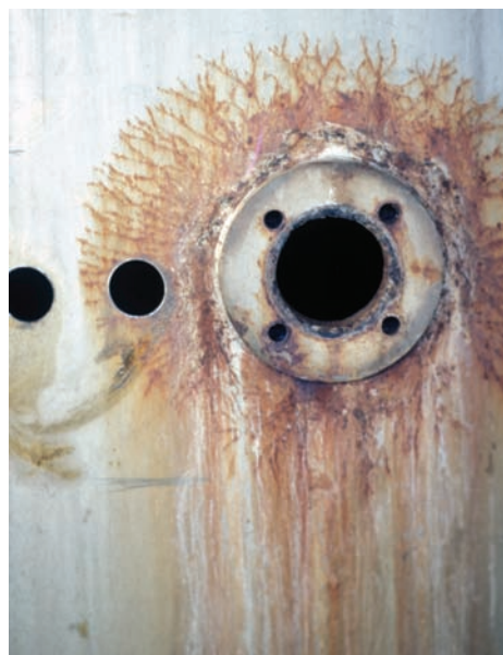
Corrosion form and mechanism Environmentally induced cracking, stress-corrosion cracking Material Type 304 stainless steel Product form Process vessel for food
