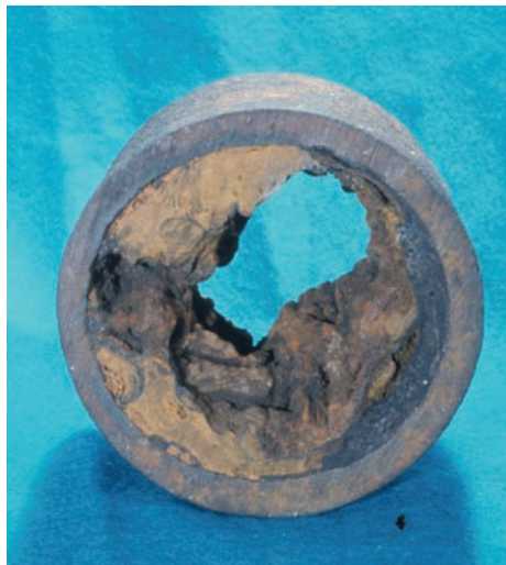
Corrosion form and mechanism Metallurgically induced corrosion, dealloying graphitic corrosion Material Gray cast iron Product form Underground mains water pipe
