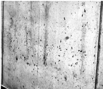
Fig. 7 Surface air voids, called bug holes , are small cavities of entrapped air bubbles in the surface of formed concrete.
