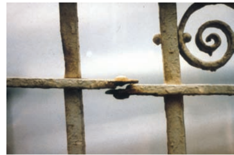
Corrosion form and mechanism Crevice and atmospheric corrosion Material Painted wrought iron Product form Guardrailing
