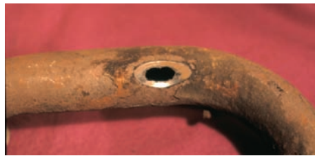
Corrosion form and mechanism Mechanically assisted degradation, fretting corrosion Material Carbon steel Product form Automotive muffler pipe
