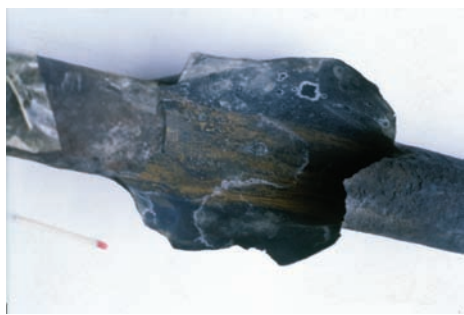
Corrosion form and mechanism High temperature, oxidation, and erosion Material Low-chromium steel Product form Boiler tube
