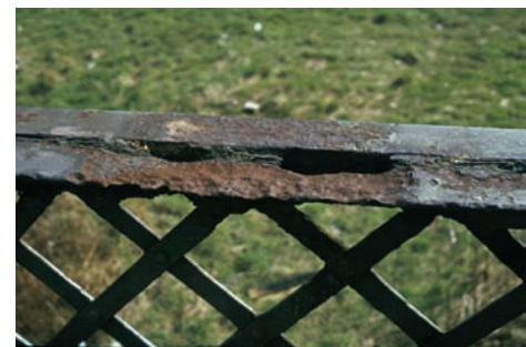
Corrosion form and mechanism Atmospheric corrosion Material Coated carbon steel Product form Footbridge
