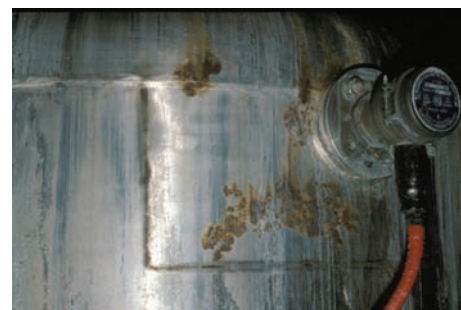
Corrosion form and mechanism Metallurgically influenced corrosion Material Type 304 stainless steel Product form Tank, food reaction vessel
