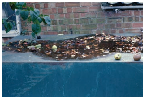
Corrosion form and mechanism Atmospheric corrosion, underdeposit attack Material Coated carbon steel Product form Oil storage tank
