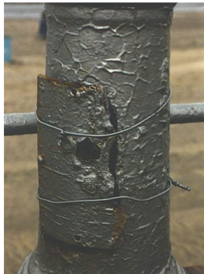
Corrosion form and mechanism Atmospheric corrosion, crevice corrosion Material Painted cast iron Product form Lamp posts
